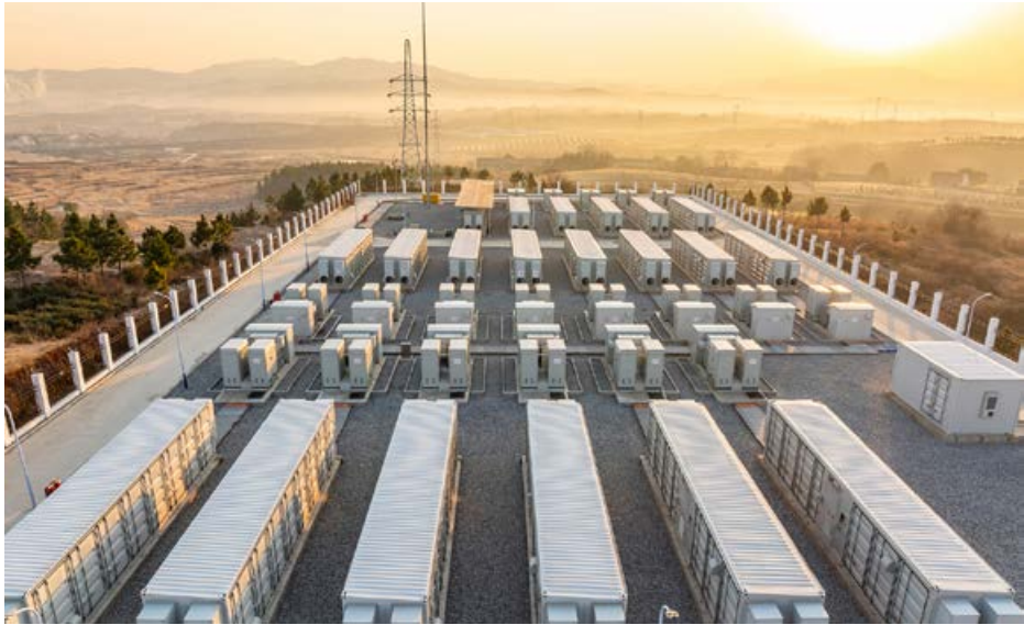
Power play Battery storage is in demand
